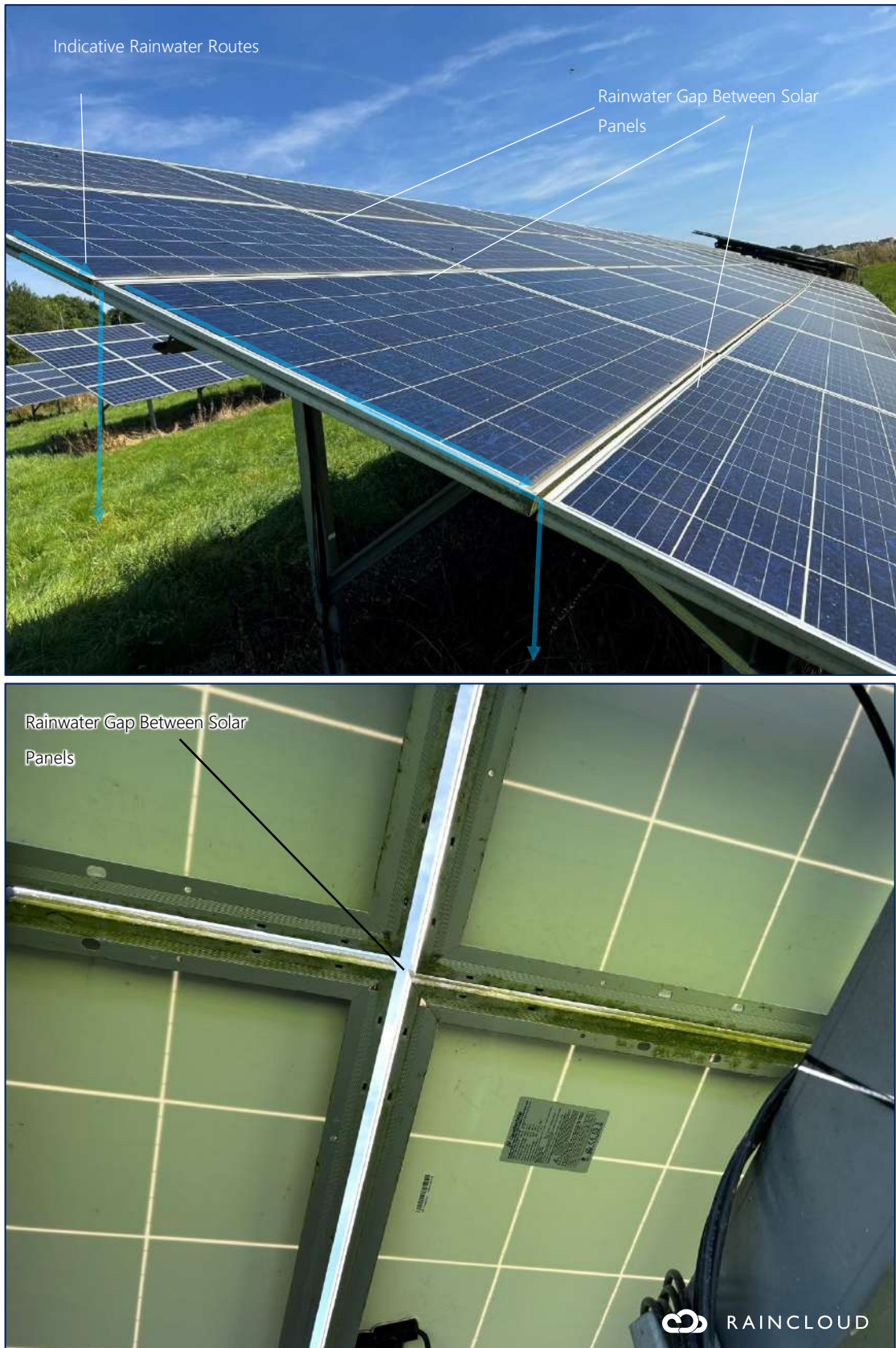
Plate 12-25 Rainwater gaps on PV array table
